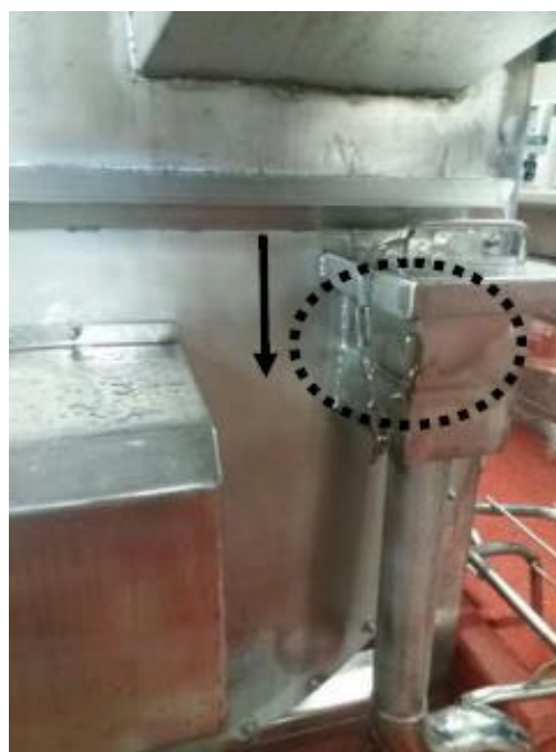
Fig. 7: Improvement in the water renewal piping of the chiller
