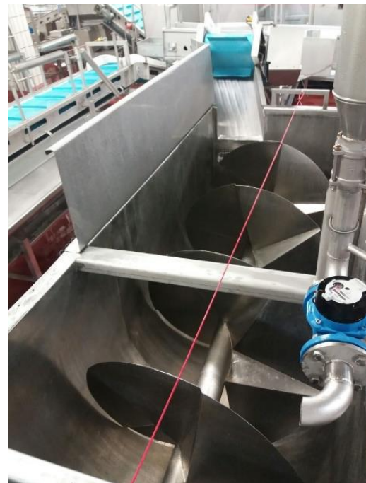
Fig. 2: Turkey leg quarter water chiller studied in this work
