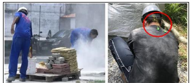
Fig. 1: Construction workers not wearing ear protectors
